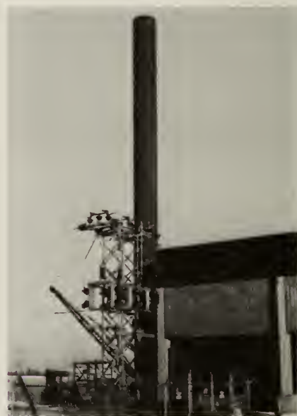
The Powerhouse supplies all the heat and electricity for the campus.
